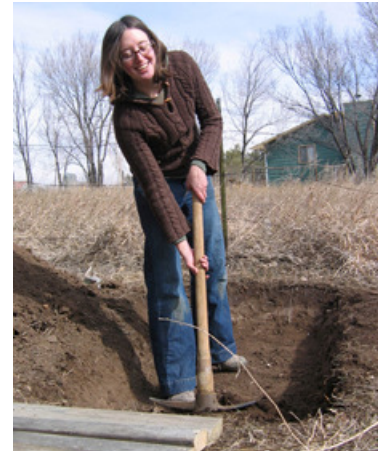
Lauren is excavating as a first step for a solar-powered electric-coil-heated hotbed ... swinging her mattock adventurously into barely defrosted February ground.
